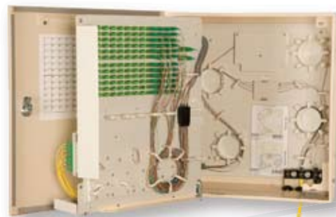
V-Linx FDH Showing Rear Panel Access
